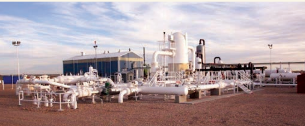
Natural gas compressor station.
