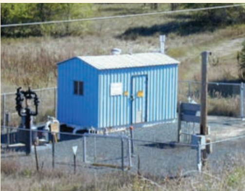
City gate meter station.
